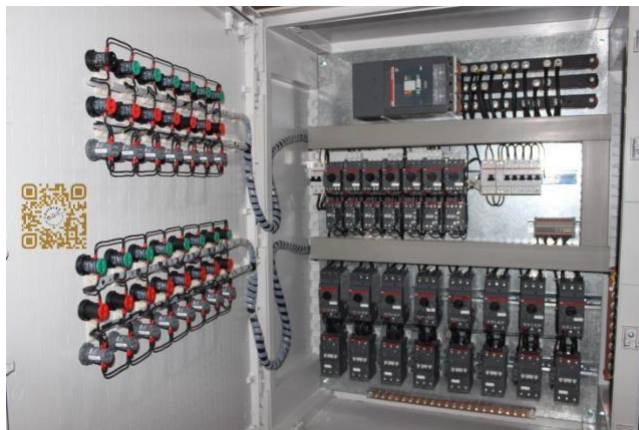
FIGURA N°5: Tablero de control CCM
